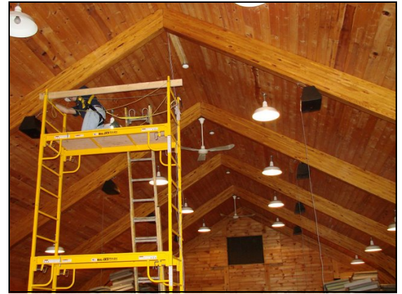
Installation of the new sound system in Newton Hall was a major project that was completed by the Association on worker's weekend.
